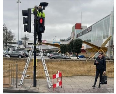
A reader sent in this snap of a uLex2 camera being installed at Brewery car park in Romford. The technician confirmed it was "for ULEZ"
